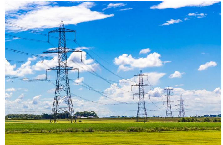
Pylons carry overhead power cables
