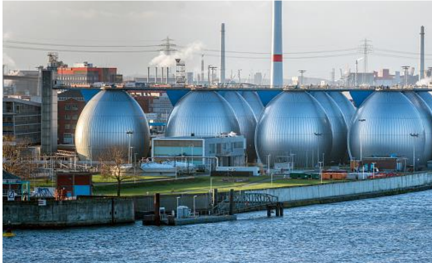
Desalination by distillation in Hamburg Germany
